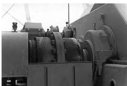
Cement kiln mill drive
